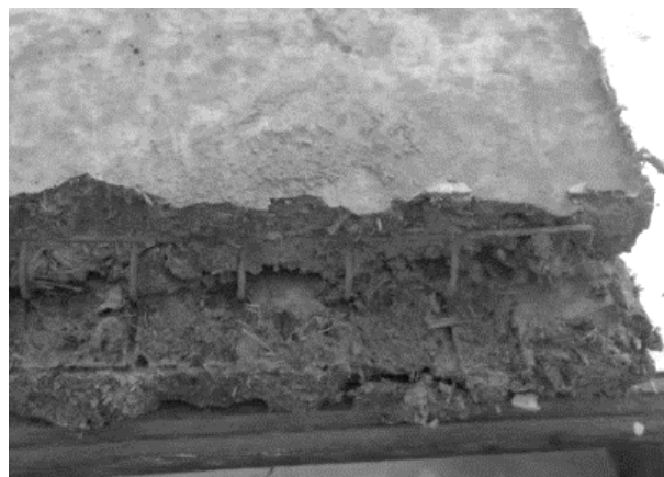
Fig. 11: Bending crack of cement board
